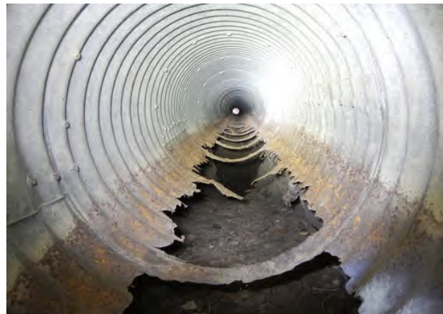
Figure 4. UAS Inspection of Deteriorated Culvert. Source: ODOT
